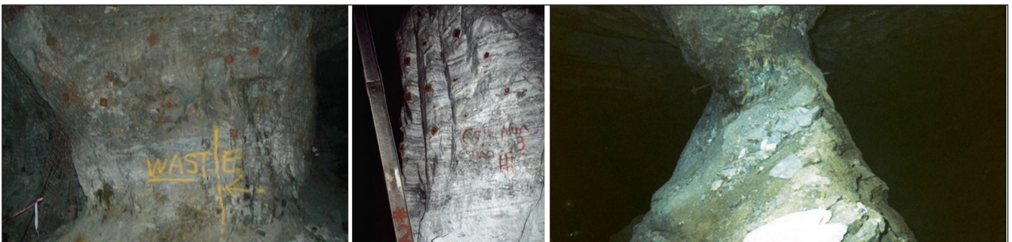
Figure 7.7 - Deterioration or change in shape pillars (such as hourglass shape with fracturing and plate-like pieces).
