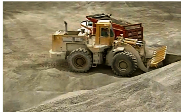
(b) Wrong - equipment angled to the face
